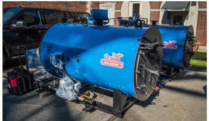
New Boilers awaiting installation
