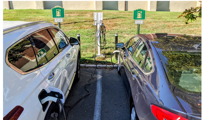
EV charging station behind the gym
